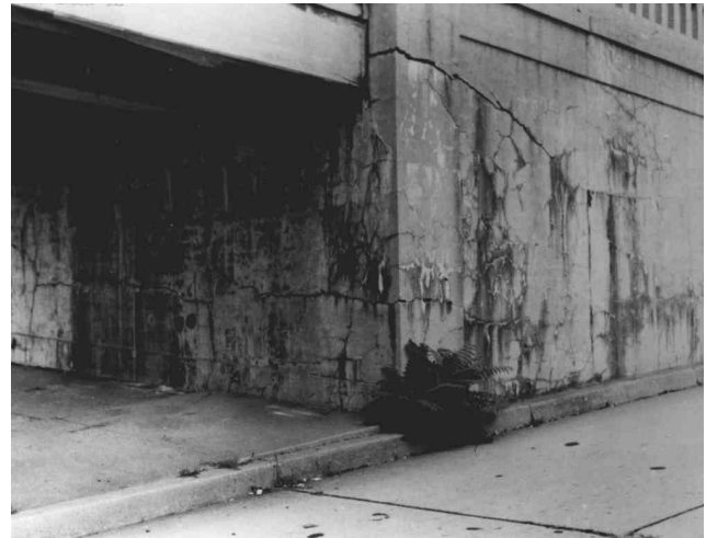
Fig. 7—Cracking caused by abnormal expansion due to alkali-aggregate reaction.
