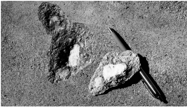
Fig. 6—Popout due to unsound aggregate particle.
